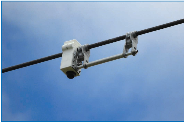
figure 12. An inclinometer installed on a phase conductor. (Source: Relogable; used with permission.)
